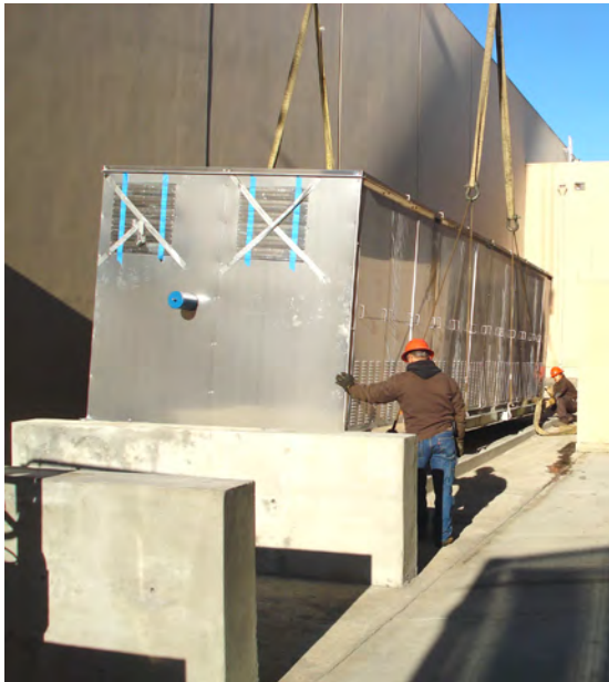
The New R507A Central Refrigeration System Houses 10 Semi-Hermetic Screw -Type Compressors For A Total Of 350 Horsepower And Is Built With An Outdoor Steel Enclosure.
