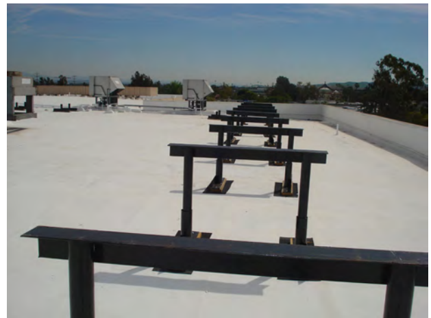
The Refrigeration Piping Is Supported With Industrial Style Steel Pipe Supports.
